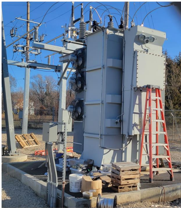
Westar (Evergy) Transformer
