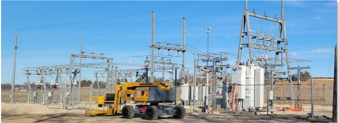
City of St. Marys Electrical Substation - 2025
