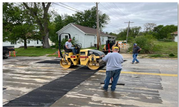
Street Department employees fixing the damage to K-63 caused by the installation of the waterline (Project 1A).
